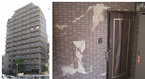
Photo.2 Residential building "A" suffered quite a heavy damage on non-structural walls. One serious problem was that the failure of such walls pushed the neighboring entrance doors and disturbed evacuation activities of residential people (2-chome, Ima-izumi, Chuo-ku, Fukuoka city).
