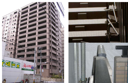
Photo.3 Residential building "B" showed pounding and suffered non-structural damage such as collapses of side-walls (the right upper) and permanent gap between two parts (the right lower). (3-chome, Yaku-in, Chuo-ku, Fukuoka city)
