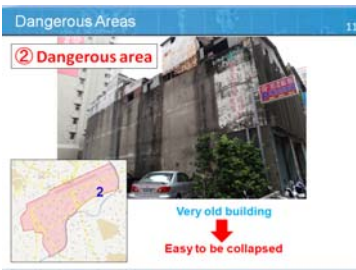
(c)危険な建物
