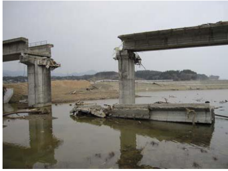
Photo 7: Fallen girder at the Sodeo-gawa Bridge (JR Kesenuma Line)
