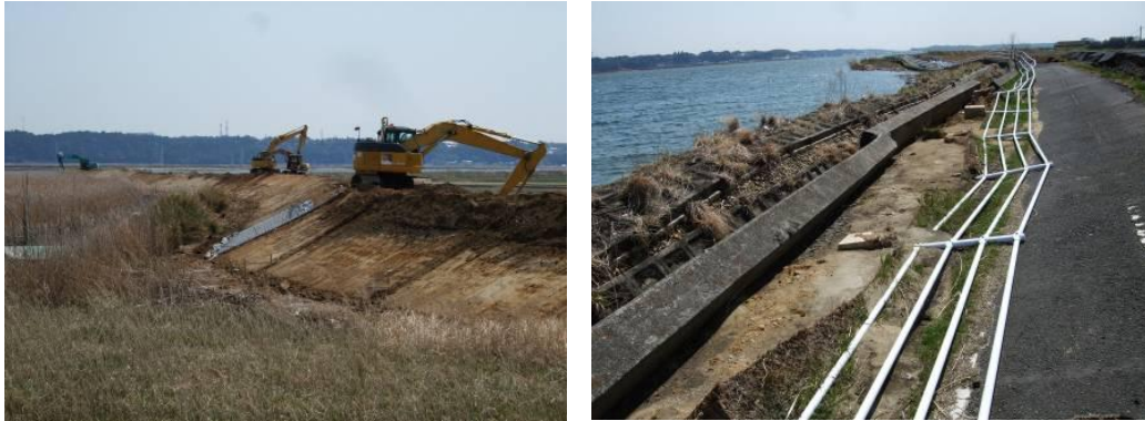
Photo 2: Levee along the Hinuma River having subsided due to its liquefaction. (At Shimoishizaki in Ibaraki town, Ibaraki Prefecture: Left Levee at River Kilometer 8.) Left view: damaged area of section under prefectural management; right view: repairs undertaken by central government. (Both April 13, 2011.)
