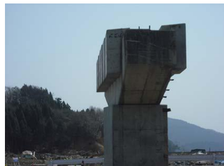
Photo 6: Anchor bars remain upright in Numata Bridge
