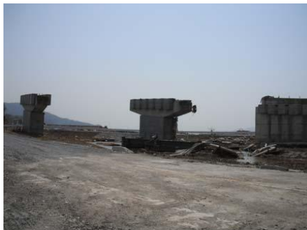
Photo 3: Numata Bridge at Rikuzentakata having lost all three main girders
