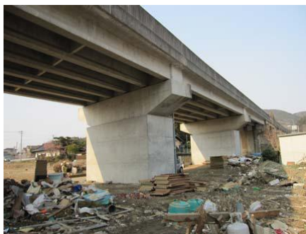
Photo 1: Intact piers of Shishiori Viaduct at Kesenuma, shown post-submersion
