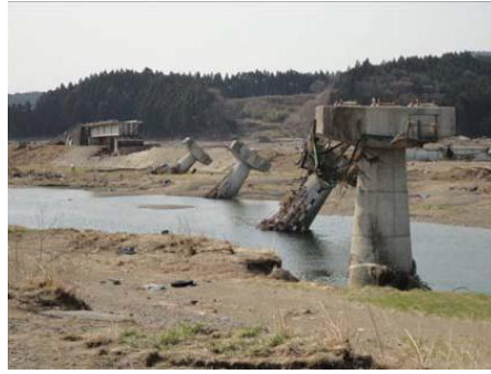
Photo 8: Collapsed piers of Tsuya-gawa Bridge (JR Kesenuma Line)
