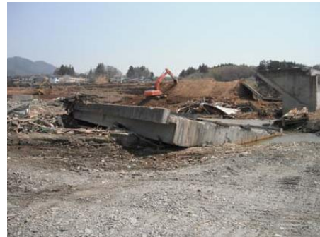
Photo 4: Fallen girders at Numata Bridge
