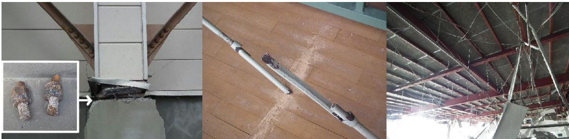
Photo 1: Column base damage at a school gymnasium
