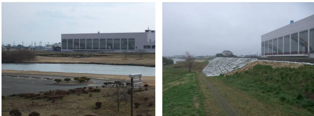
Photo 1: Levee along the Eai River having subsided due to liquefaction of its foundation (At Furukawa-Fukunuma in Osaki City, Miyagi Prefecture: Right Levee at River Kilometer 26.8). Left: before repairs (view from opposite bank, March 14, 2011); Right: after restoration (April 22, 2011)
