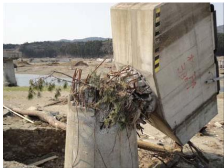
Photo 9: Broken pier of Tsuya-gawa Bridge (JR Kesenuma Line)
