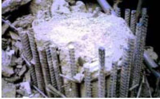
Fig.10 Lap splices failure of rectangular Column
