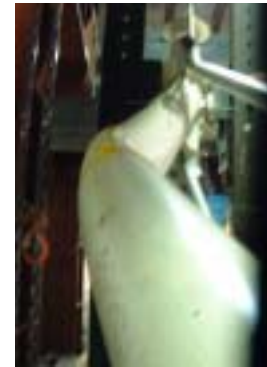
Figure 13(c) Diagonal buckling
