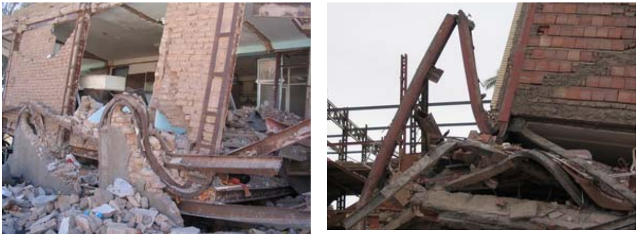
Figure 16 Folded columns caused by the vertical component of the earthquake.
