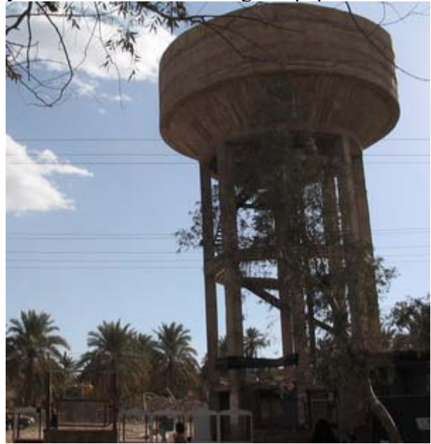
Figure 17 The Bam's elevated water tank and the cracking of its concrete cover at joints . As it can be seen from the picture, smooth steel bar has been used as the re-inforement .
