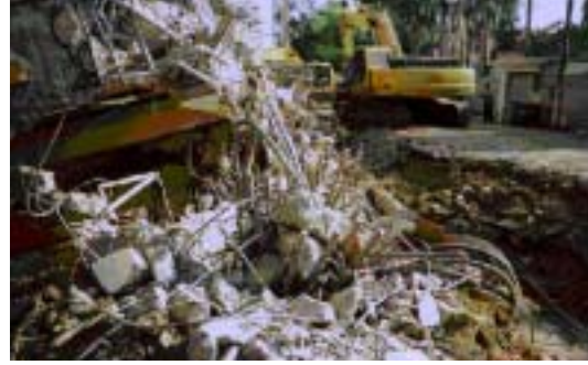
Fig.11 Lap splices failure in a collapsed building
