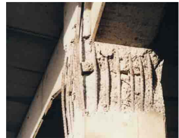
Photo.12 Failures of the top of columns in JR (Nishinomiya)
