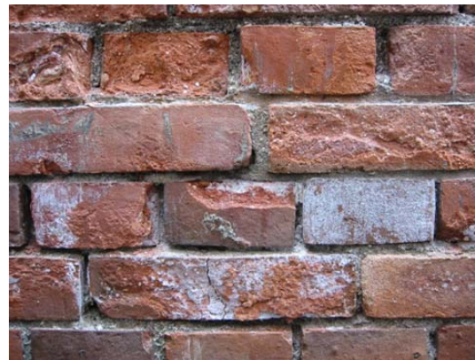
Figure 3 Spalling caused by crystalline salt residue inside the brickwork
