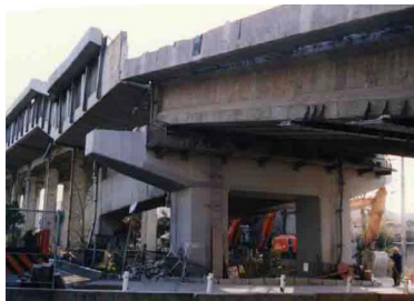
Photo.11 JR-Shinkansen with heavy Beams and columns (Nishinomiya)
