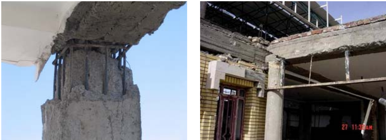
Figure 13 Concrete structures without required hoop spacing or proper beam-column connection details.
