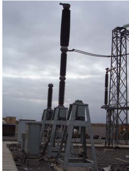
Figure 19 The damages inflicted to the city's only substation.
