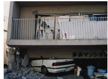
Photo.3 Soft first story suffered heavy damage in many places (Motoyama, Kobe)
