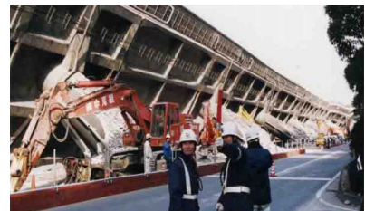
Photo.6 Overturning failure of Hanshin Highway (Fukae, Higashinada, Kobe)
