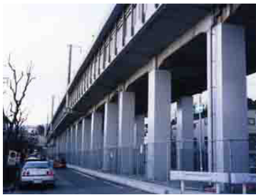
Photo.13 JR-Shinkansen after temporary repairs (Nishinomiya)
