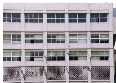
Photo.16 One directional shear failure of a school building (Okamoto, Kobe)
