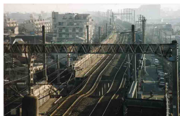
Photo.5 Failure of JR-Super Express called Shinkansen (Nishinomiya)
